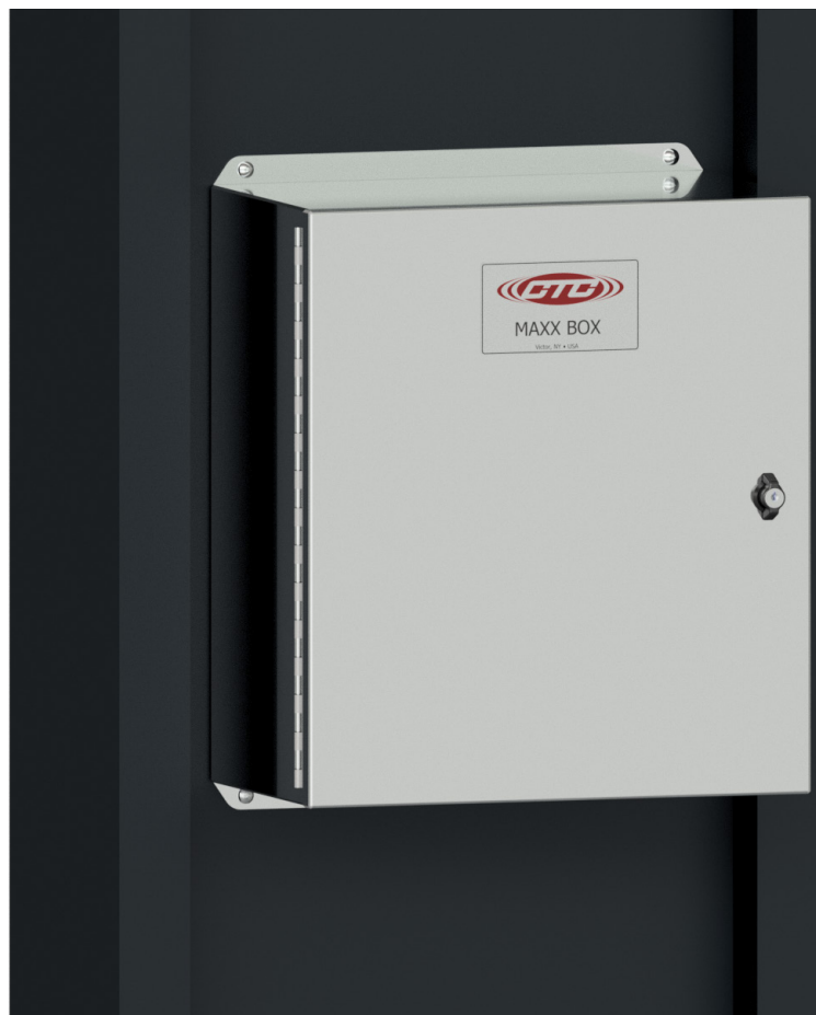
Figure 5. Switch Box (MX433) Earth Ground
