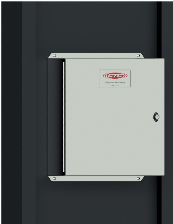
Figure 5. Switch Box (JB230) Earth Ground
