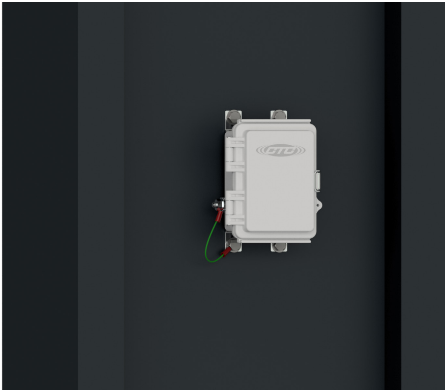
Figure 5. Termination Box (MX704) Earth Ground
