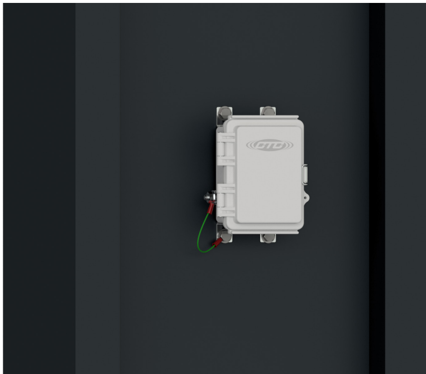
Figure 5. Termination Box (MX702) Earth Ground
