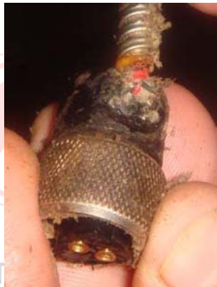
Figure 1; Improperly specified polycarbonate connector showing deterioration two years into service.
