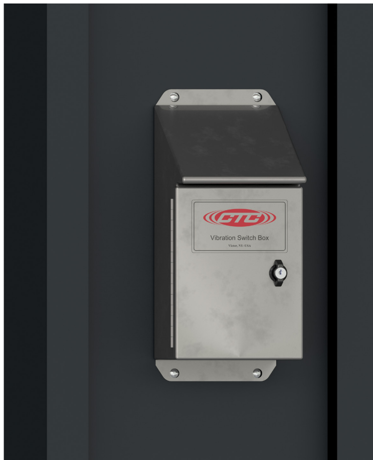
Figure 5. Switch Box (SB262) Earth Ground
