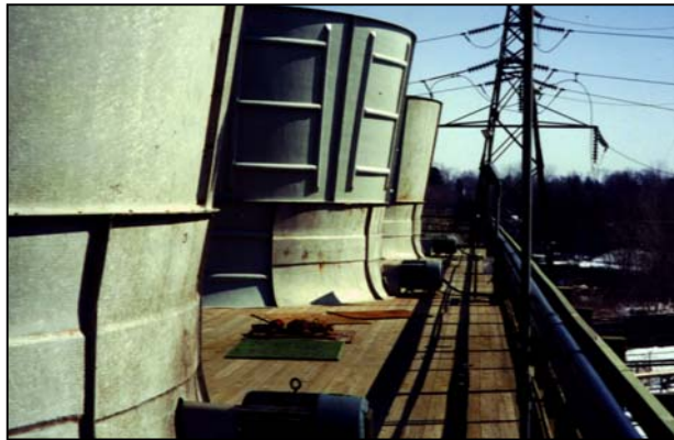
Cooling Towers assist in maintaining plant operating temperatures.
