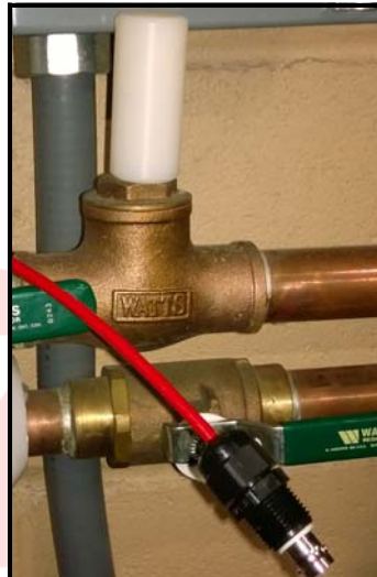
Figure 4— EMPP with cover removed, ready to take data. Note cover resting on check valve in the background.
