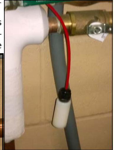
Figure 3— EMPP with cover in place.
