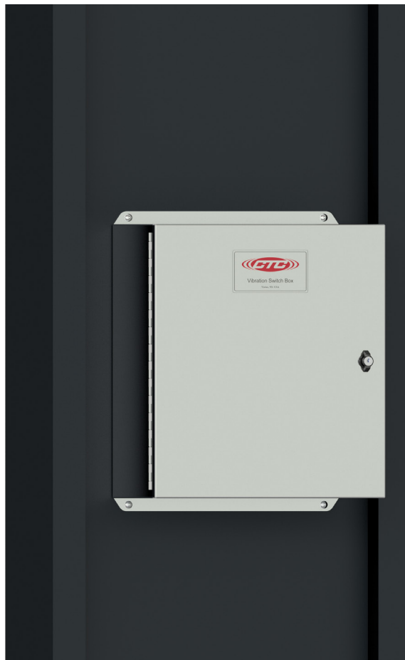
Figure 5. Switch Box (SB202) Earth Ground
