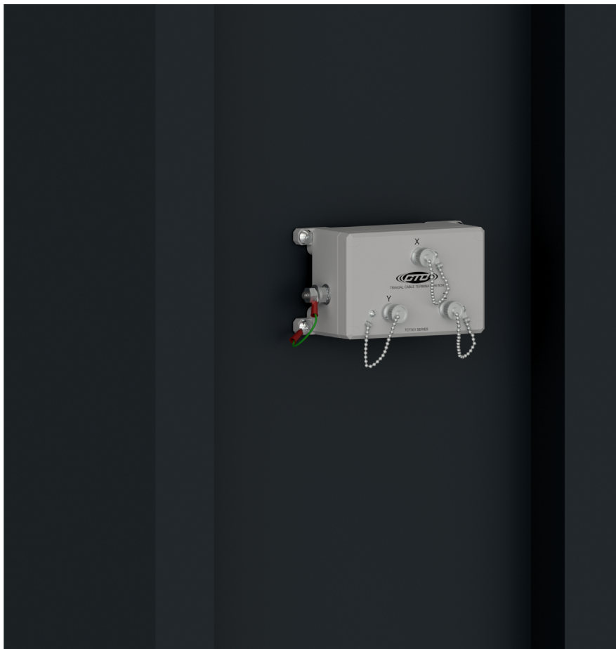
Figure 5. Cable Termination Box Earth Ground
